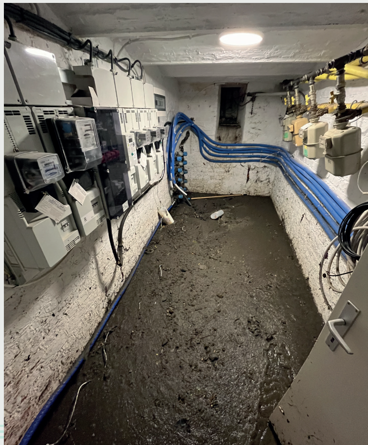
Figure 3: Flooding in the basement of one of the households affected (Resident, July 9 2024)
